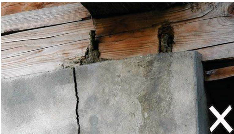
RCC column fixed to timber beam. This is not permitted.
