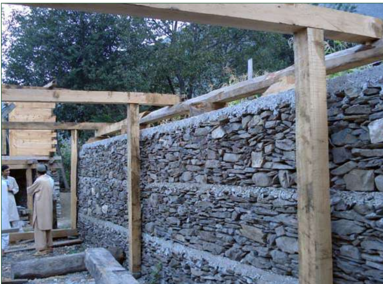
Timber posts inside and separate to the wall. RCC bands between well laid dry stone masonry.
