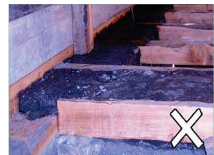
Heavy insulation in the roof is dangerous.
