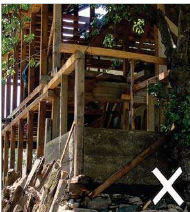
Even small areas of in situ may weaken the frame.
