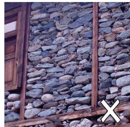
Stonework with no bracing.
