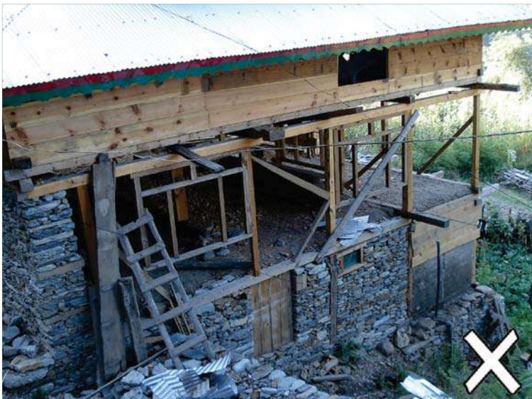
More than 1 storey retaining wall. Plan area not same for each storey.
